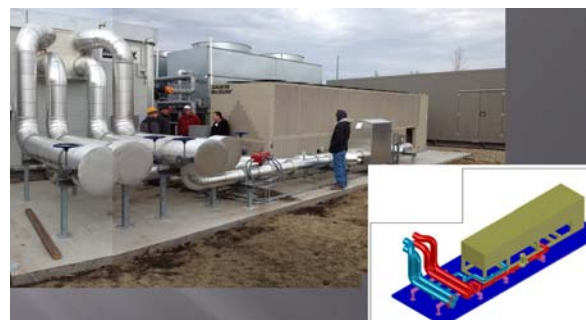
Air Cooled Pathfinder Chiller (Above)
