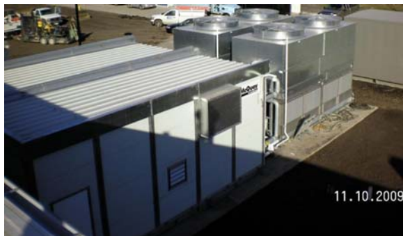
Modular Central Plant (Above)
