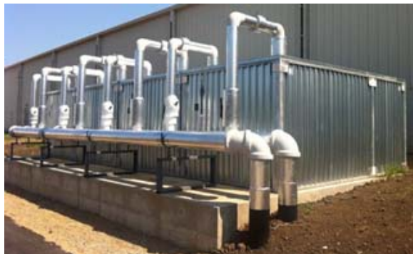
FAFCO Ice Storage, utilizing underground piping to yield a clean appearance (Above)
